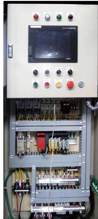
■ Control devices (Control panel)
