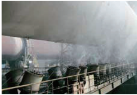
Industrial cooling system
