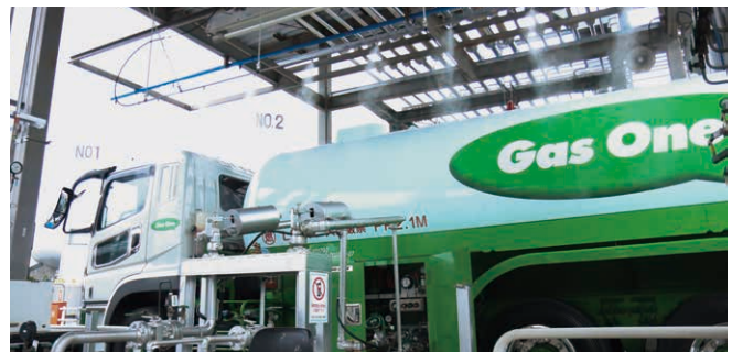
▲Mist cooling system also installed the tank truck station
